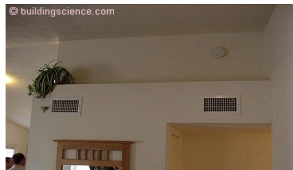
Photograph 3: No Short Circuiting - The supply duct and the return duct could be located up high on the same wall a couple of feet apart.
