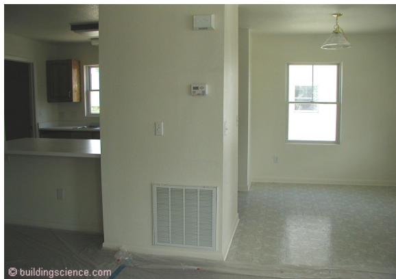
Photograph 7: Single Return - The single return at the main floor level has an “offset” to handle blower noise.
