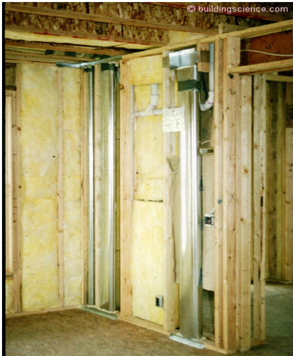
Photograph 1: High Supply Registers - As window thermal performance improved, we learned to “throw” the air across the room from registers located high on interior walls.
