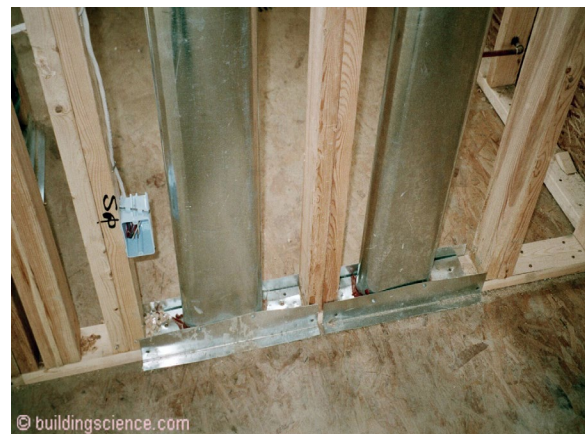
Photograph 2: Small Ducts - Better windows also meant smaller ducts. Ducts could easily fit in interior walls.
