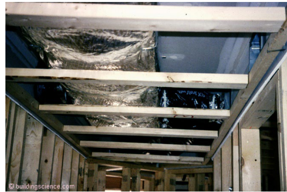
Photograph 8: Dropped Ceiling – Ductwork located in a hallway/corridor dropped ceiling. The supply and returns are in the same dropped ceiling.
