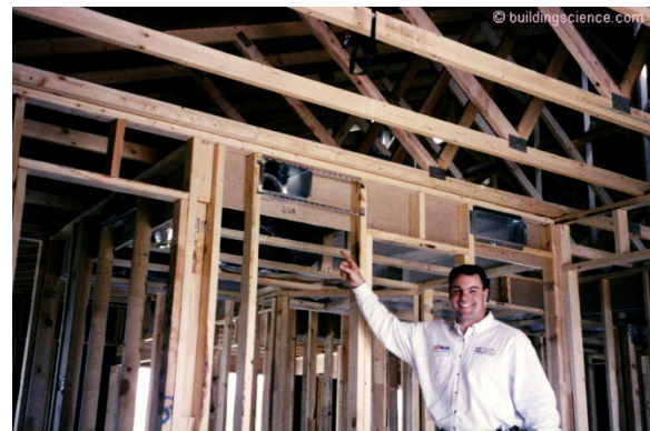
Photograph 10: Still More Dropped Ceiling - The supply grilles and return grilles share the same wall.
