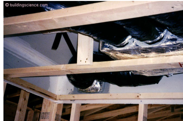
Photograph 9: More Dropped Ceiling - The returns are "passive" – transfer grilles into the dropped ceiling and a large ceiling register in the corridor dropped ceiling connecting the dropped ceiling to the corridor. The supplies are "active" hard ducted.
