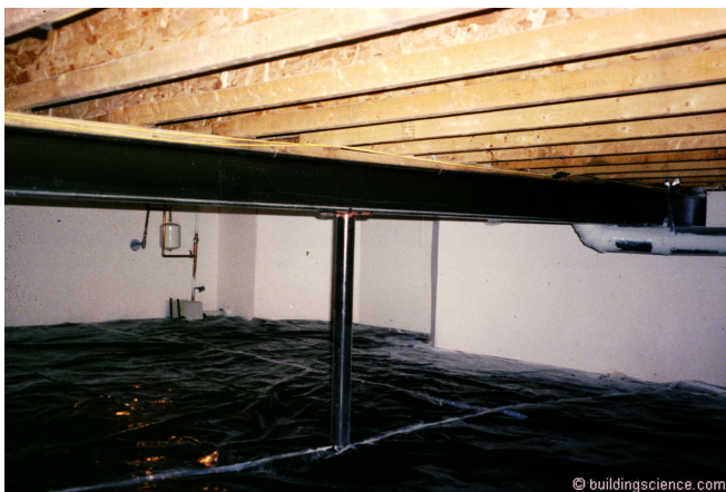
Photograph 3: Conditioned Crawlspace – The way crawlspaces should look. Dry, warm, part of the house, not part of the outside or part of the ground. Insulated on the perimeter not in the floor. Beautiful.
