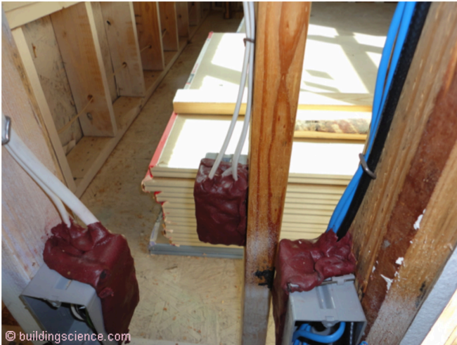
© buildingscience.com Photograph 5: Airtight Electrical Box – putty pads are used to seal electrical boxes airtight. Joint compound is used to complete the seal between the electrical box lip and the cut opening in the gypsum board.
