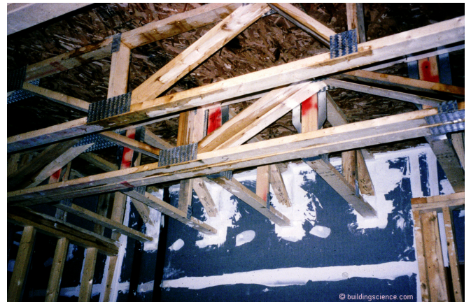
Photograph 3: Compartmentalization Air Sealing – gypsum board is run up to the underside of the floor sheathing above and sealed with joint compound.
