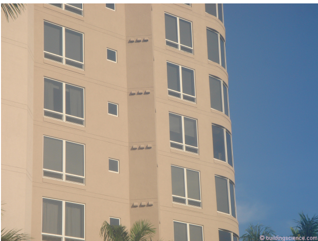
© buildingscience.com Photograph 7: Penetrations in Exterior Walls – yes, there need to be more of them.
