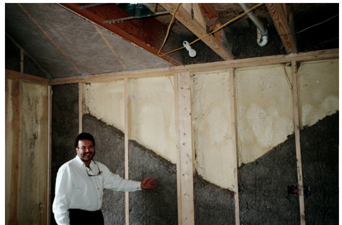
Photograph 1: Hybrid Wall Assembly Legend – Jay Epstein proudly presenting his hybrid closed cell spray polyurethane and damp spray cellulose wall before it became "fashionable"...Not going to give you the date of this photograph...but the hair color is not that dark anymore....
