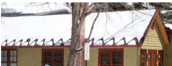
Photograph 3: Heating Cables —Throw energy at the problem. Heating cables are still a pretty common approach to dealing with ice dams.
