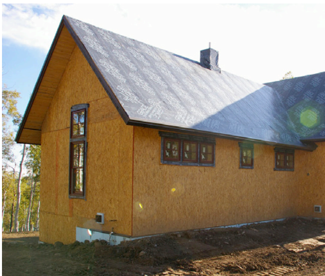
Photograph 4: Insurance —It is not uncommon to install a water protection membrane on the entire roof to keep ice dam melt water out of roof assemblies. This does not prevent the ice dam from occurring; it only limits the damage.
