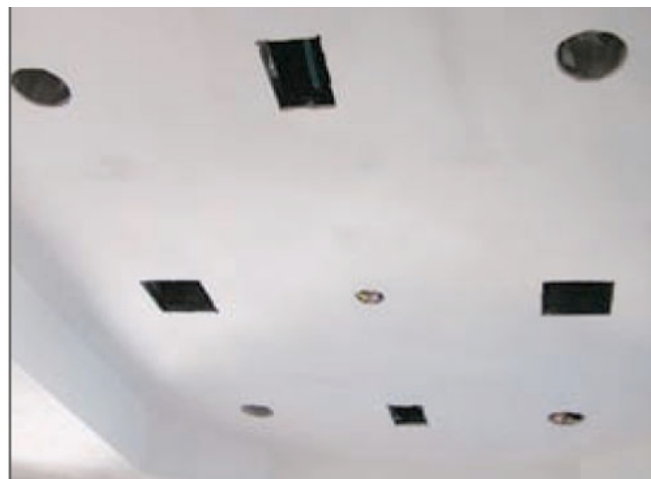
Photograph 5: Swiss Cheese Ceiling —Can you believe the perforations we put in attic ceilings? What are the odds that each one of these is going to be sealed airtight? Right. When they leak air, they leak heat, and the heat warms up the roof deck, and that is a problem. Air leakage induced attic heat gain is far more of a concern than conductive and radiative attic heat gain. In other words, airtightness is more important than insulation levels. But both are important.
