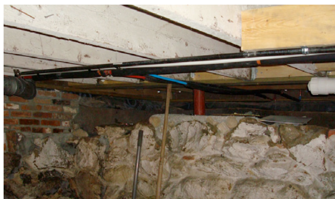
Photograph 2: Knocking Out the Demising Wall —Note the small short column that replaces the supporting demising that was removed to connect the crawlspace to the house basement.
