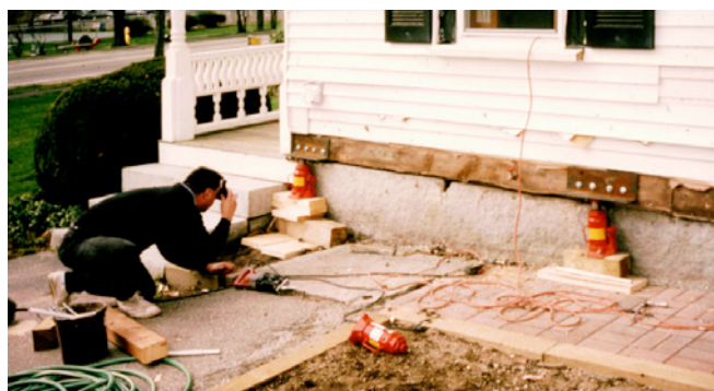
Photograph 3: Disbelieving Neighbor —Yes, you can actually lift a house off its foundation a section at a time with small hydraulic jacks and steel angles lag bolted into the bottom of the timber frame. We used 5 jacks rented from the local hardware store—three on the outside approximately 10 to 12 feet apart and two on the inside at the lifting mid points to keep the timber rim beam from rotating. A membrane capillary break was installed between the top of the rubble wall and the timber frame.
