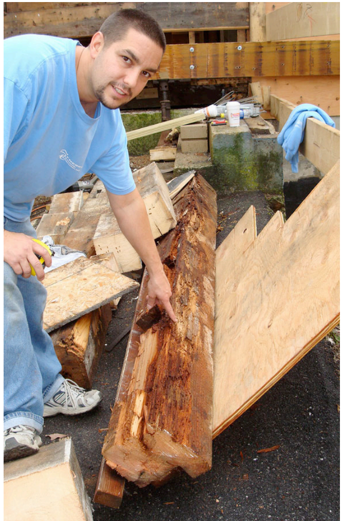
Photograph 11: Rotted Bearing Timbers —Many of the bearing timbers typically have to be replaced due to serious rot.
