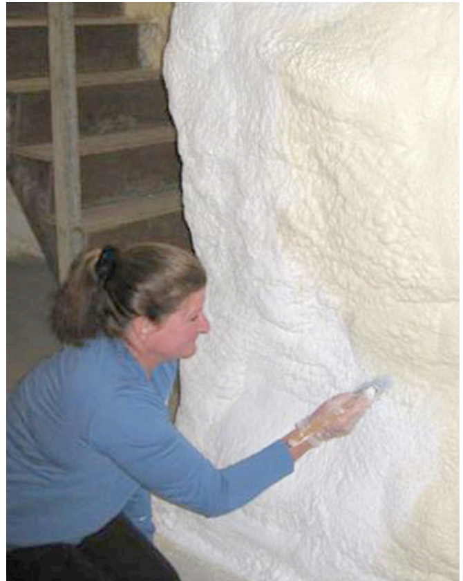
Photograph 8: Intumescent Coating —A liquid applied ignition barrier is recommended as minimum protection for exposed spray foam. I think that perhaps a bigger brush would have made it go faster – just a thought.
