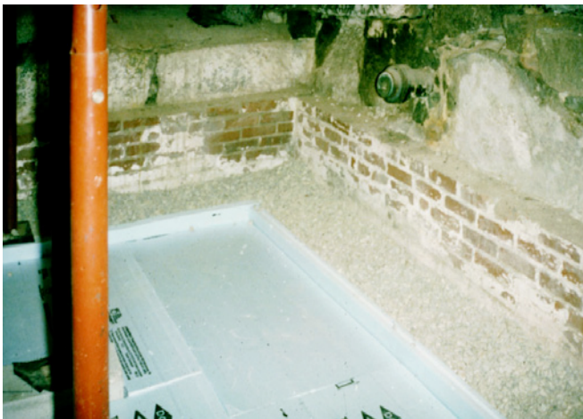
Photograph 4: Foam Bathtub —Extruded polystyrene foam on top of a gravel layer on top of the existing combination dirt and broken concrete slab floor. The perimeter drain was located in the space between the foam “bathtub” and the perimeter foundation wall in the granular layer perimeter drainage zone. A new concrete slab was cast inside the foam “bathtub.”
