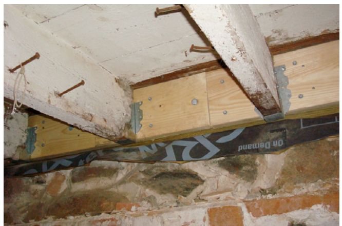
Photograph 12: Rebuilding Sill Assembly —Bolts and hangers and more bolts and hangers and still more...
