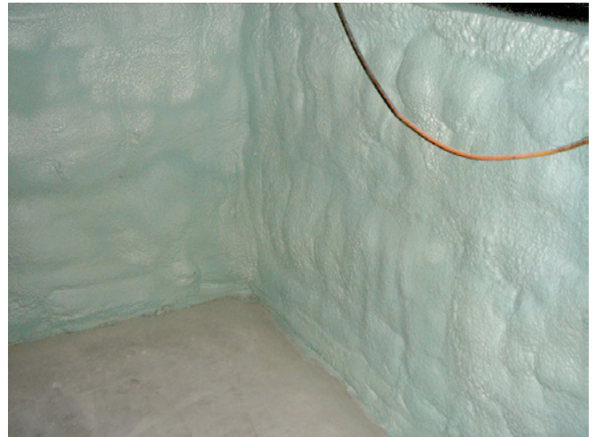
Photograph 14: Spray Foam Layer —The foam itself is “structural” in that it is rigid enough to support itself if it is between 2 and 3 inches thick and if it adheres to the wood frame at the top of the foundation (which it does) and if it adheres to the edge of the foam bathtub at the bottom of the foundation (which it does).
