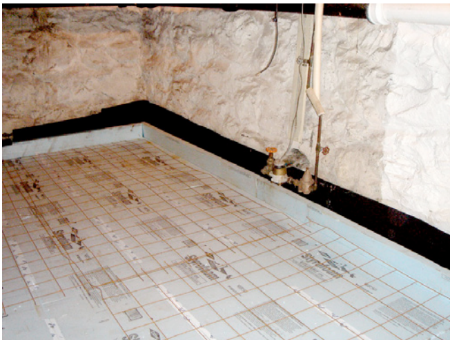
Photograph 13: Another Foam Bathtub —Note the “twist” in the approach. The cleverness of this detail is that a granular drainage layer under the foam insulation and “yet-to-be-cast” slab has been replaced with a ¾-inch drainage mat that extends up the walls about a foot. The ¾-inch mat does what 4 inches of stones used to do.
