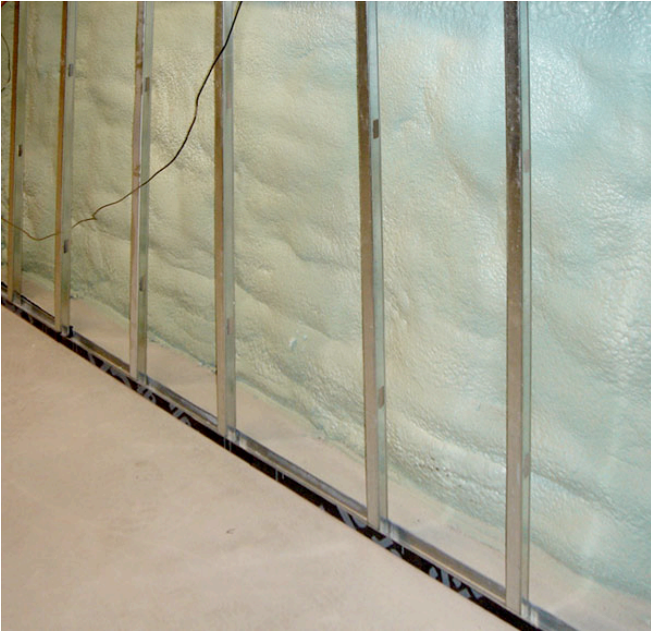
Photograph 16: Protection for Insulation Layer —As nice as the foam is to look at it really should be protected from mechanical damage and from ignition sources. That's where thin lightweight steel framing and gypsum board are ideal.
