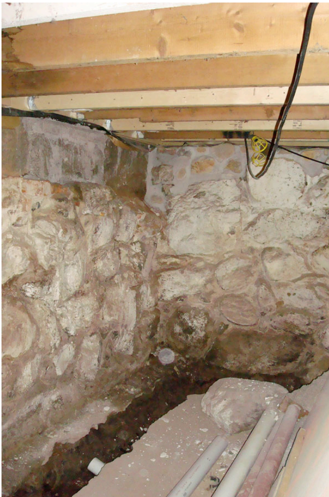
Photograph 9: Trenching For Perimeter Drain —Most rubble foundations have very thin and weak ground slabs – if they are anything at all besides dirt – that are easy to break through with simple tools such as a pick, a pike and sweat.
