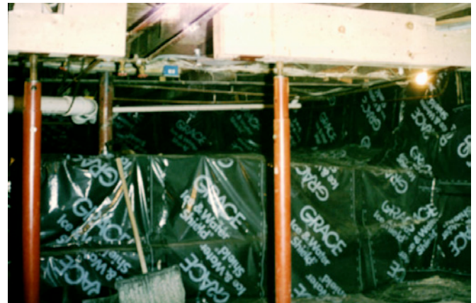
Photograph 5: “Pool Liner” —A sheet polyethylene butyl composite membrane lining was installed covering the interior perimeter rubble foundation wall and the upper short crawlspace floor. This membrane lining was sealed to the capillary break that was installed on the top of the rubble foundation under the timber frame and also sealed to the new concrete slab cast inside the foam “bathtub.”
