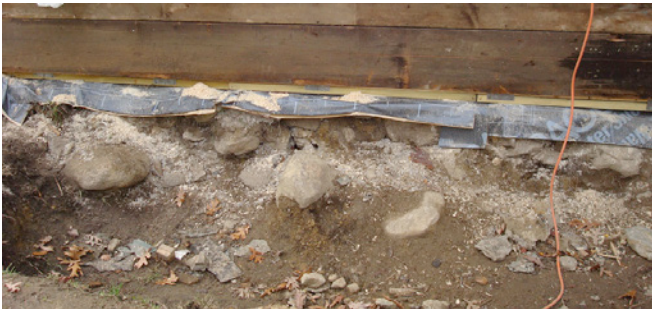
Photograph 10: Capillary Break Critical —Many rubble foundations do not project much above grade. The installation of a robust capillary break is a necessity along with lowering the immediate adjacent grade.
