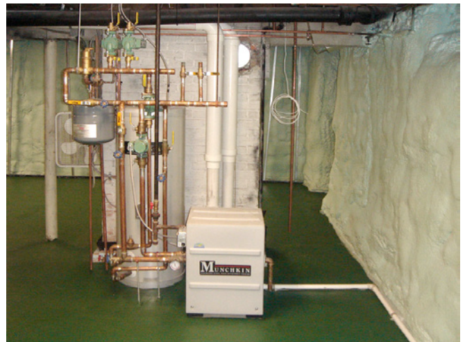
Photograph 15: Mechanical Equipment —Very nice home for some very happy mechanical equipment. This equipment is best when it is sealed combustion and power vented as the old air leaky foundation is now pretty much airtight.
