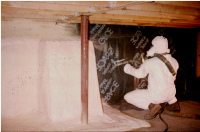
Photograph 6: Insulation Layer —The interior surface of the membrane lining was insulated with direct spray applied polyurethane foam – the high density closed cell stuff.
