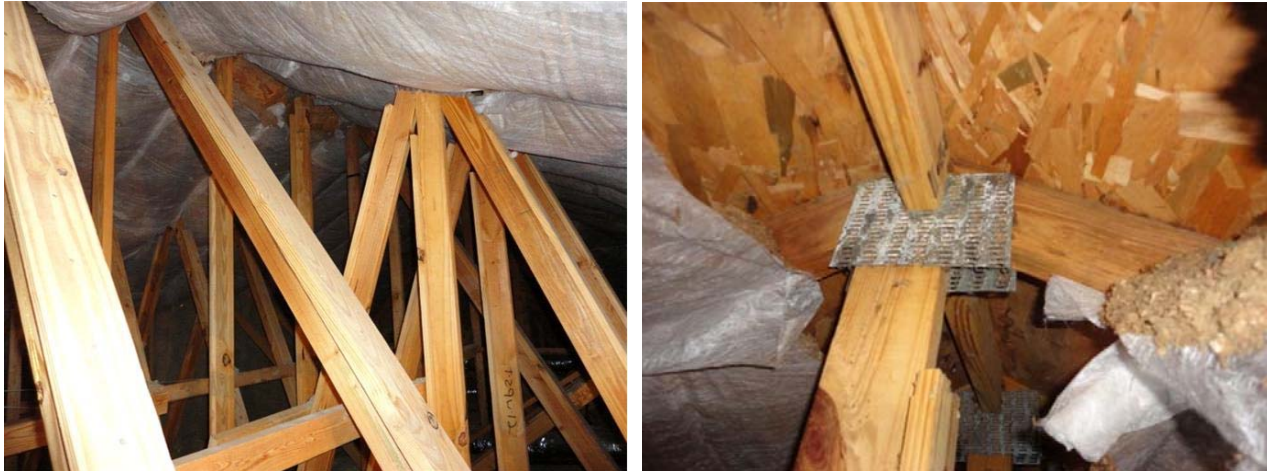
Figure 10. Cellulose roof insulation in Jacksonville (left); corrosion of ridge truss plate (right)
