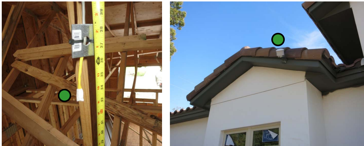
Figure 31. Typical temperature/RH sensor for attic interior (left) and exterior (right) conditions
