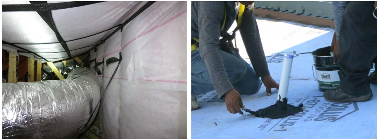
Figure 20. Insulated attic knee wall (left) and waterproofing/air barrier at roof penetration (right)
