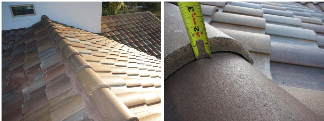
Figure 26. Completed roof ridge tile geometry (left); gaps in ridge tile (right)
