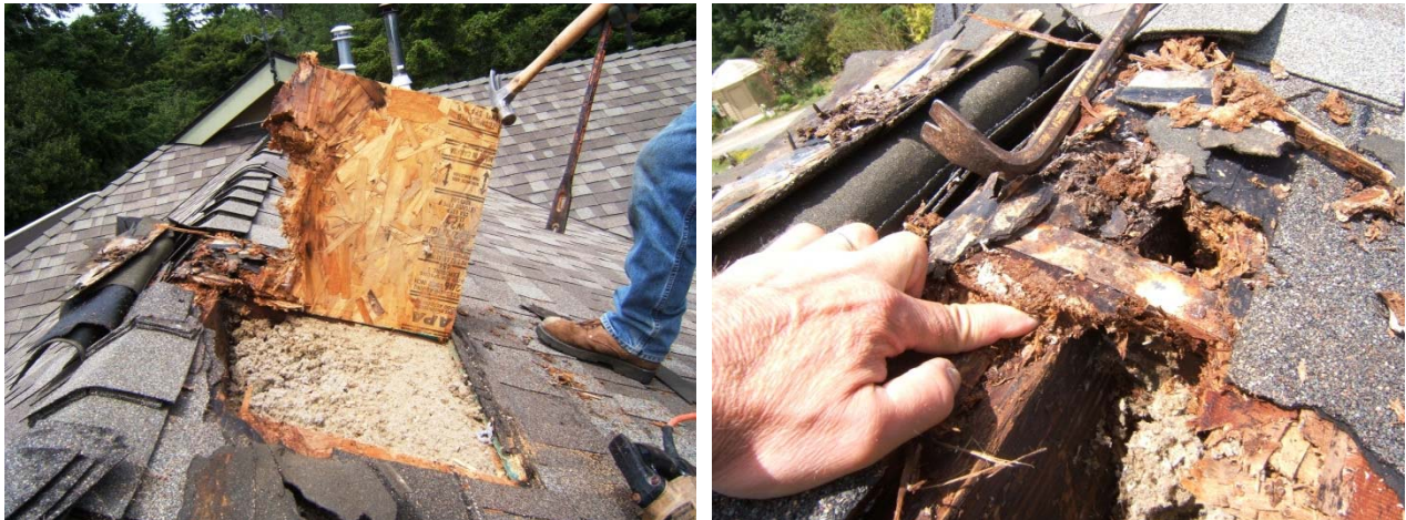
Figure 11. Ridge sheathing degradation with dense-pack cellulose in northern California
