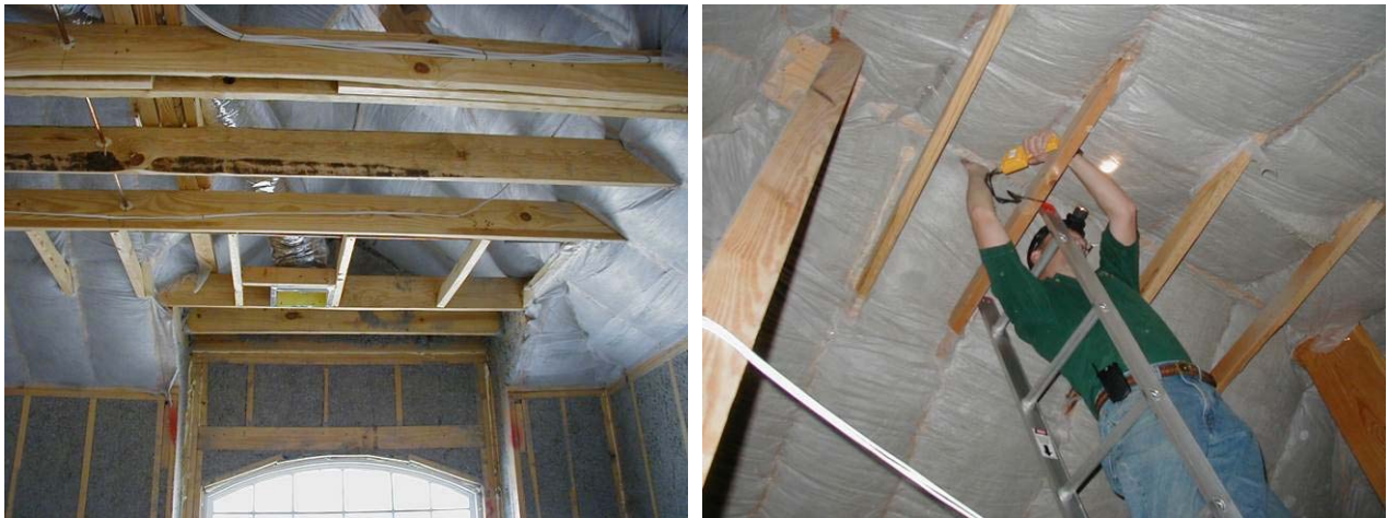
Figure 9. Netted and blown cellulose roof insulation in Houston (left); MC at the roof ridge (right)
