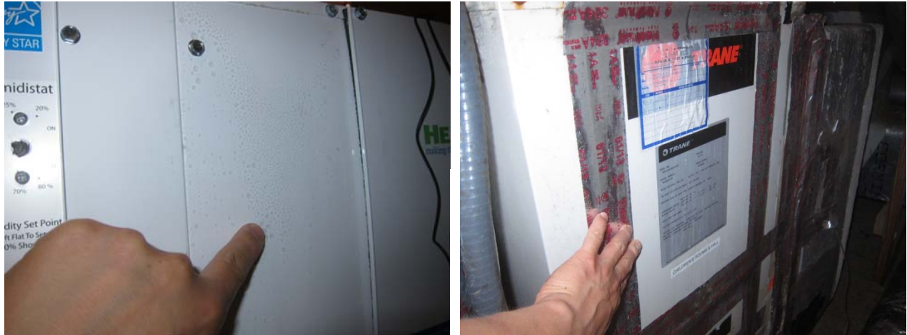
Figure 5. Condensation on HVAC equipment located in vented attic (CZ 2A)
