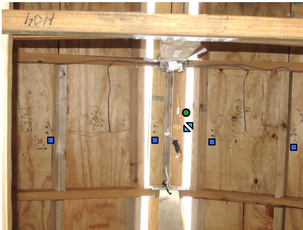
Figure 29. Typical ridge monitoring package with sensors highlighted
