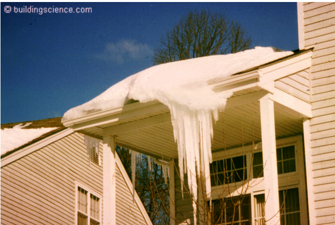
Photograph 6: Classic Ice Dam – Can be prevented and controlled with ventilation.
