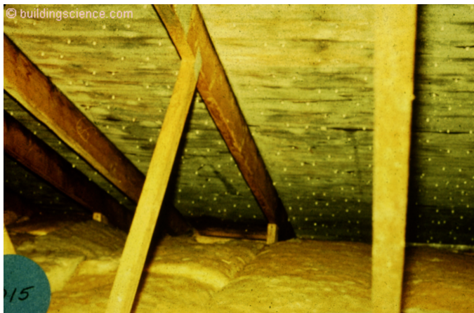
Photograph 2: More Roof Rot – Frost on nails and roof sheathing.
