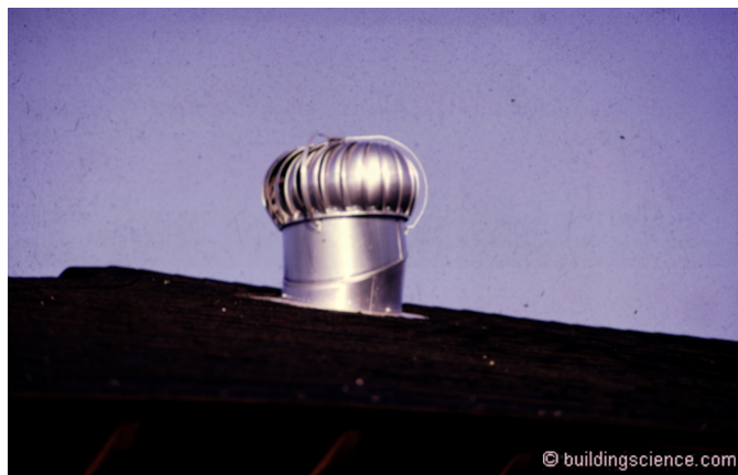
Photograph 4: Turbine Vents – Typically lead to increased air conditioning bills.
