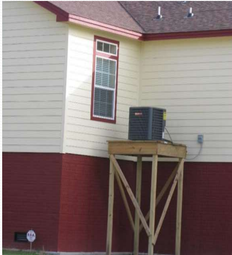
elevated A/C unit
