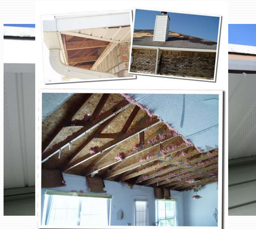
Suspended soffit vents
