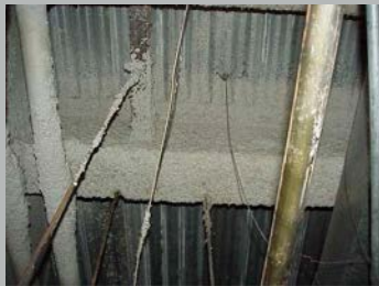
Sprayed-on fireproofing material
