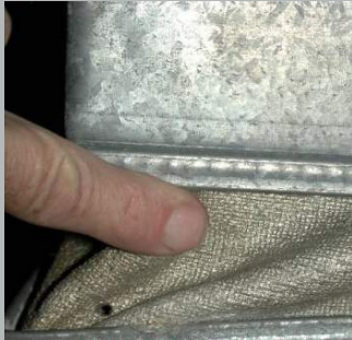
Asbestos fabric in HVAC system
