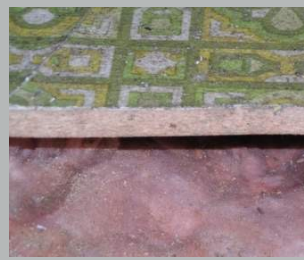
Sheet vinyl containing asbestos
